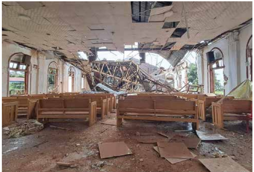
The interior of a Christian church in Chin State after a military attack, one of a series of assaults on civilian infrastructure protected under international humanitarian law. Photos: CHRO
