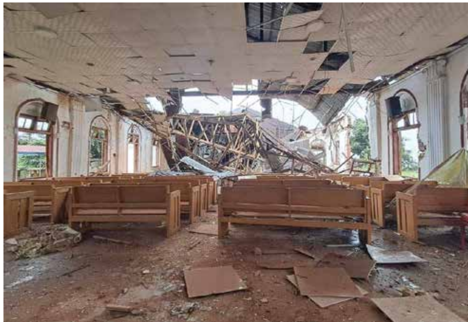
The interior of a Christian church in Chin State after a military attack, one of a series of assaults on civilian infrastructure protected under international humanitarian law. Photos: CHRO
